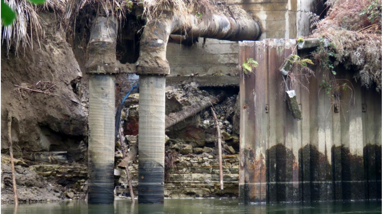
Figure 5. Photograph showing failure of sheet pile wall and erosion extent
