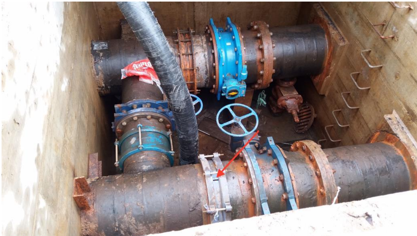
Figure 4. Photograph showing exact location of gibault failure once isolated
