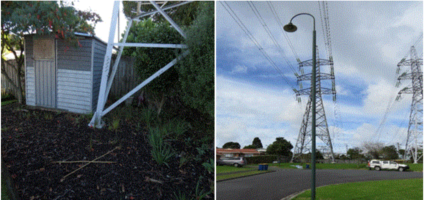
Photograph 2: A power line tower located adjacent to a gardening shed is connected to other towers via an overhead earth wire that is also parallel to another power line
