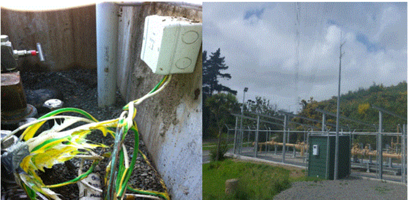
Photograph 1: Examples of melted Cathodic Protection (CP) cable insulation caused by LFI and pipeline telemetry equipment damaged by a power line EPR
