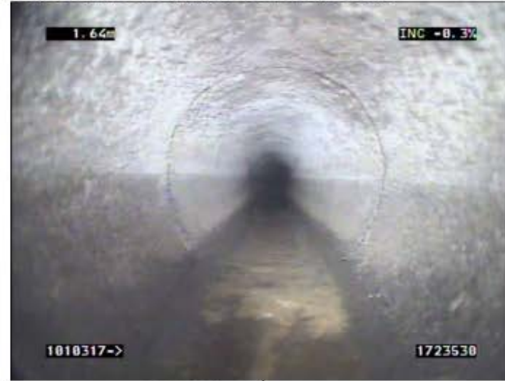
3.2m General Observation - Corrosion to 9mm
