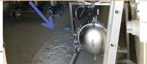
CHLORINATION SYSTEM IN PRE CAST CONCRETE BUILDING. 70KG CHLORINATION GAS SYSTEM WITH V-NOTCH MOTORIZED VALVE, PANEL HEATER AND WEIGH SCALE!
