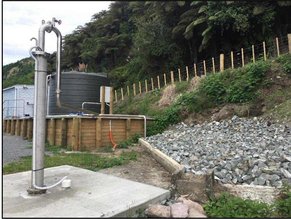
Photograph 5: Tahuna Road WTP after Upgrade
