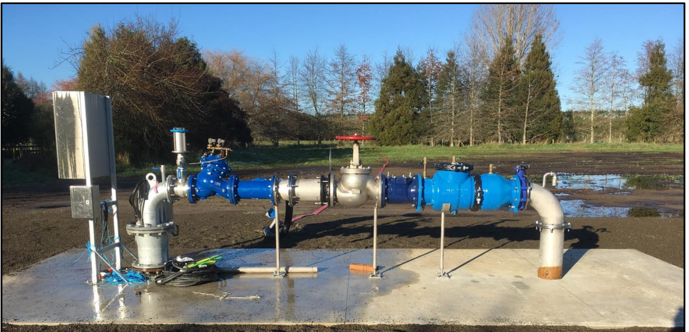
Photograph 3: Bore Head pipework.
