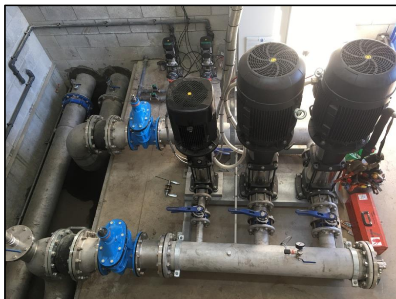
Photograph 4: Booster Pump and Manifold
