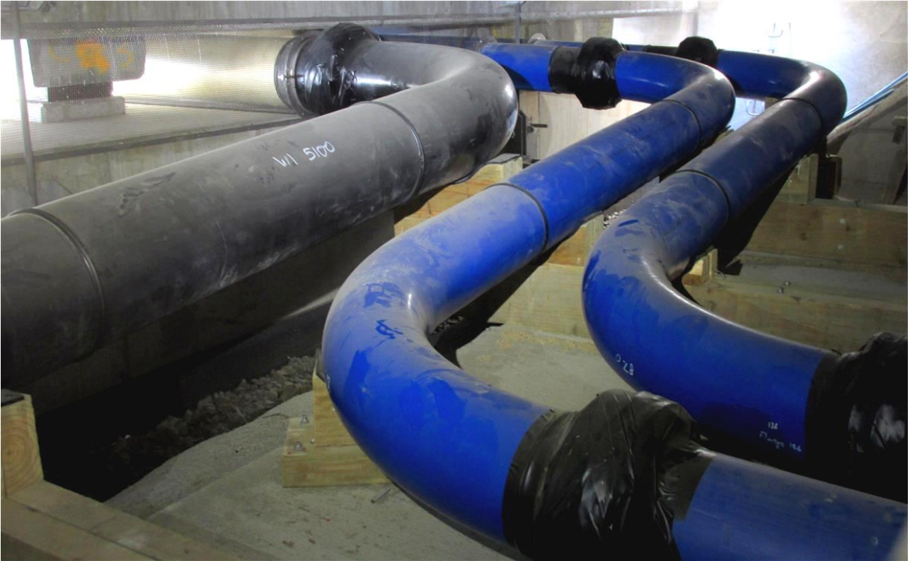
Photograph 1: View of the installed "cranked" specials on the City side of the river. The DN 450 sewage pressure main crank has been extruded from black PN 16 PE 100 resin.
