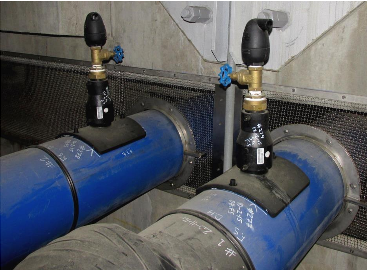
Photograph 2: View of the air valves on the DN 355 water mains on the Sumner side of the river. The stainless steel mesh prevents unauthorized access to the cavity area.
