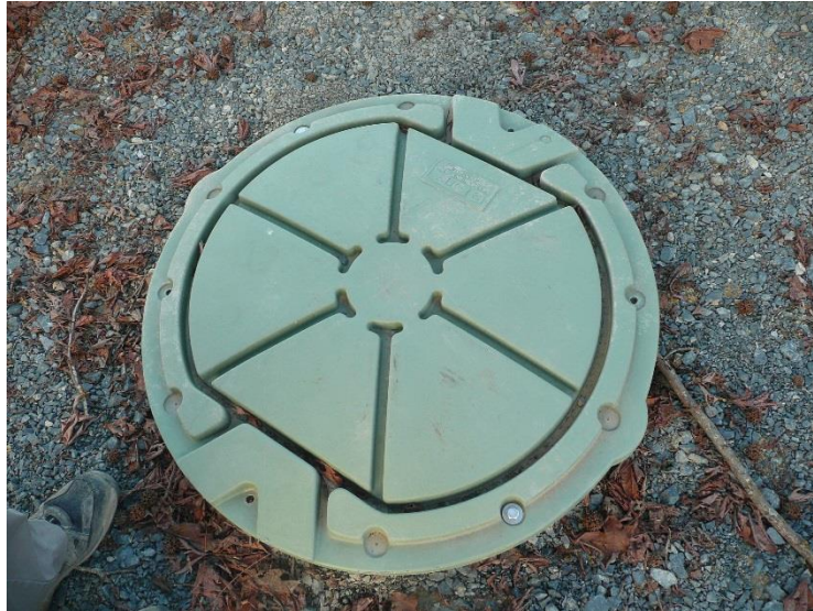
Photograph 2: A recently installed Pressure Sewer Chamber in private property
