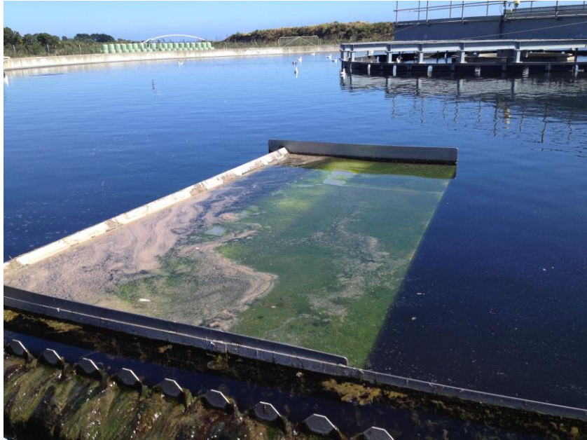
Figure 1: Photo of Wet Scum Beach on Secondary Clarifier at New Plymouth WWTP.
