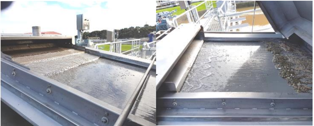
Figure 7: Photographs of Baleen Filter (with hood up) During Scum Dewatering operation.
