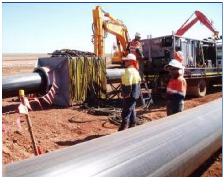
Figure 6. Reducing the diameter of the HSCR PE100 liner pipe prior to insertion.
