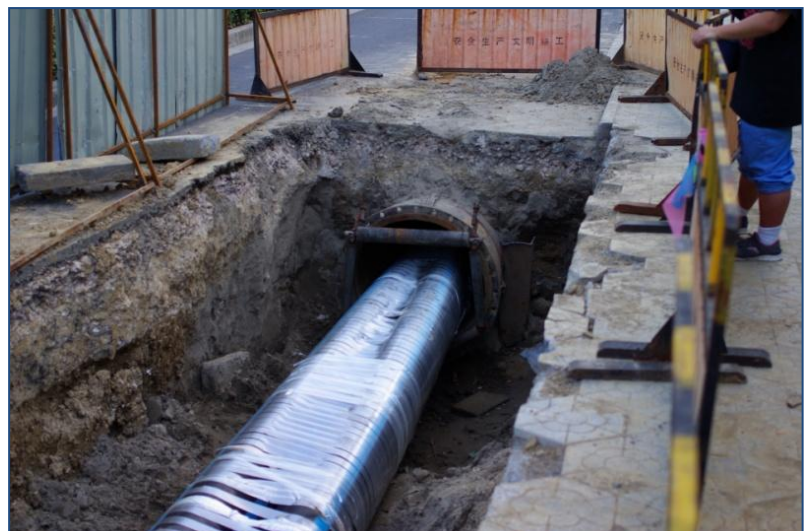
Figure 7. The pipe folded and strapped being inserted into the old leaking water main
