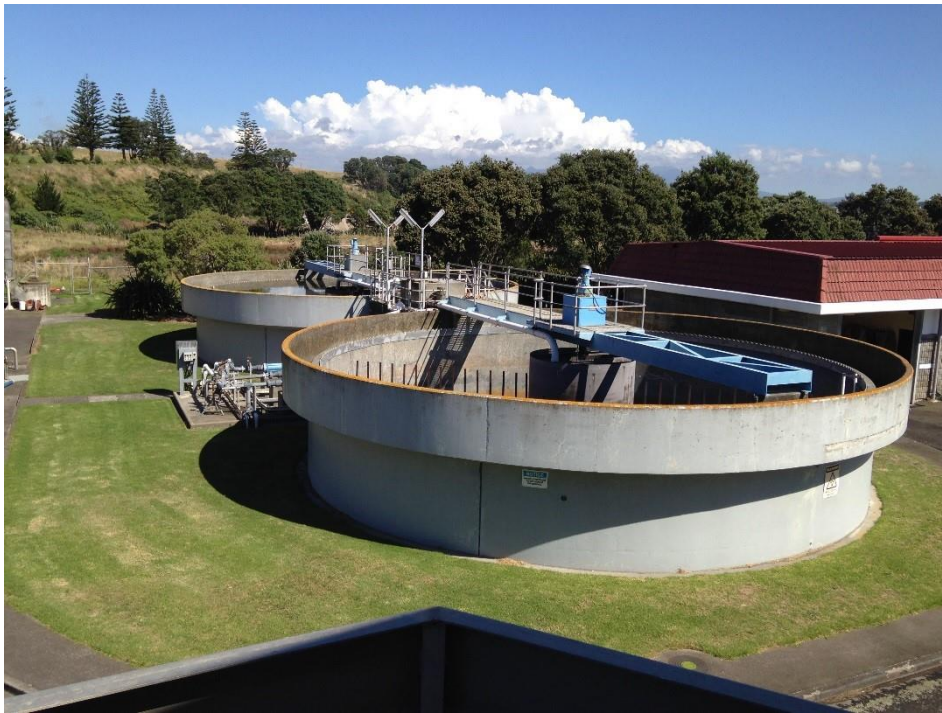
Figure 1: Aerial View of Two Picket Fence Thickeners at New Plymouth WWTP, Prior to Upgrade.
