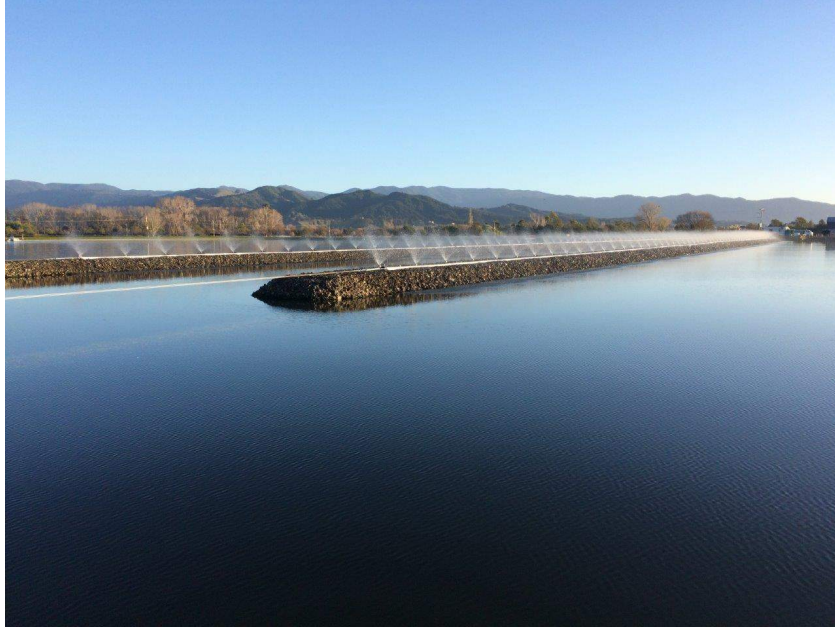
Photo 1: Rock nitrification sprays at Motueka WWTP
