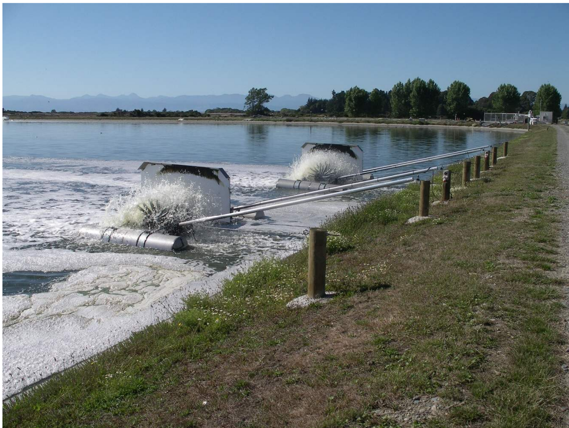
Photo 4: Pond 2 Brush Aerators
