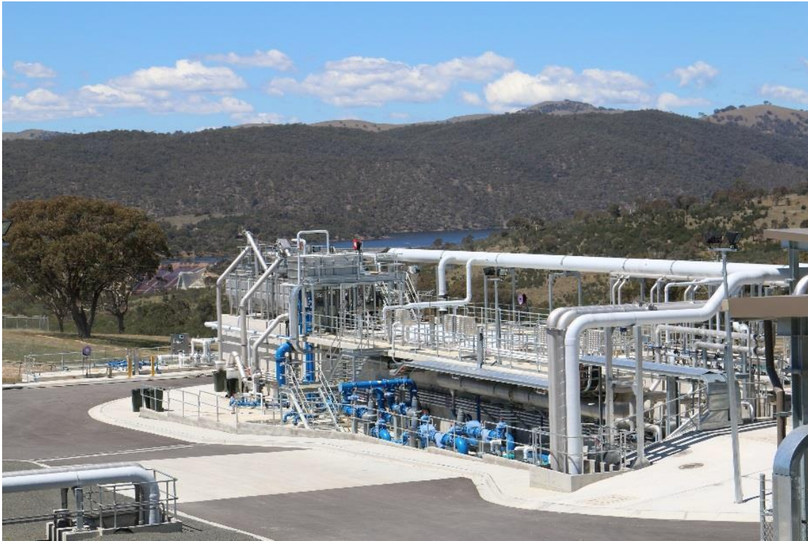
Photograph 1: Membrane bioreactor at the Googong Water Recycling Plant
