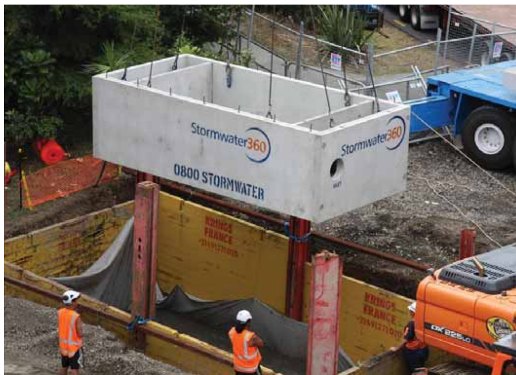
Below – Stormwater360’s StormFilter vault being lowered into place by crane, Bottom – Lid being installed to complete a StormFilter vault
