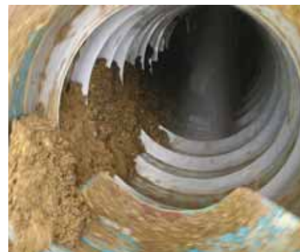
Above – ROTO-SIEVE in action, Top – ROTO-SIEVE High Performance Drum Screens in an MBR Plant
