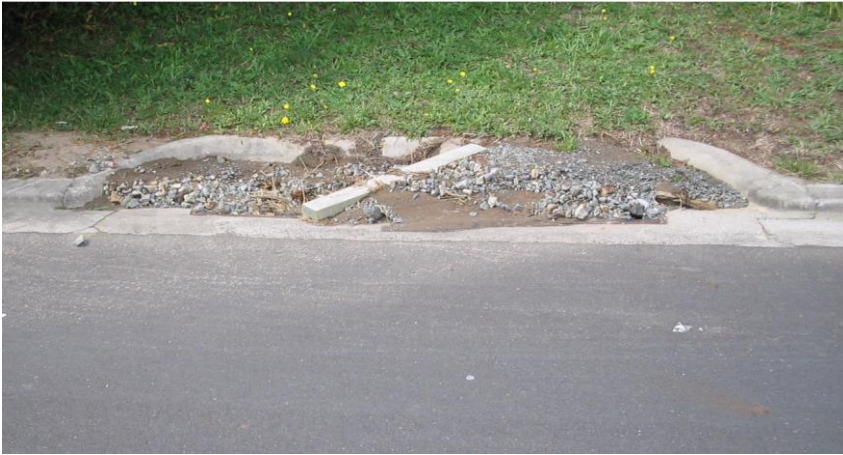
Figure 4 – an example of double sump blocked with silt, gravel and debris (courtesy of Eric Thorn, Opus)
