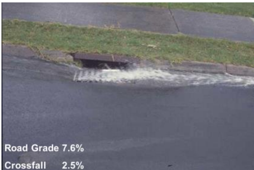
Figure 3 – two examples of sumps being by-passed by flow from a hydrant test (courtesy of Eric Thorn, Opus)
