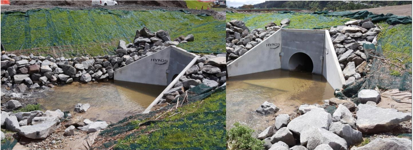
Figure 9: Photographs showing the debris line following the November 2016 storm event
