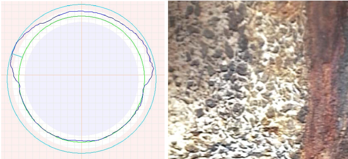
Figure 5 – Laser profile of 450mm wastewater pipe after 40 years (Clearwater Systems 2010)
