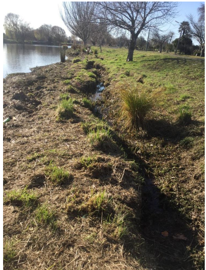
Photograph 2: Example of severe earthquake damage to unlined waterway
