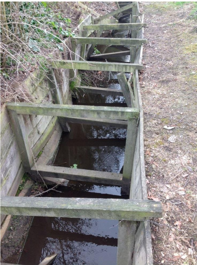
Photograph 1: Example of severe earthquake damage to timber lined drain
