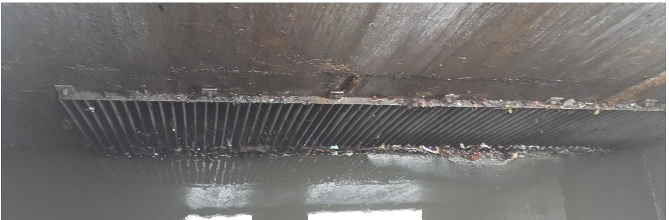
Figure 3: Existing silt well bar screen (50 mm spacing).
