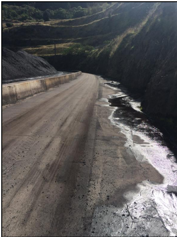
Photograph 2: Contamination on the existing concrete road
