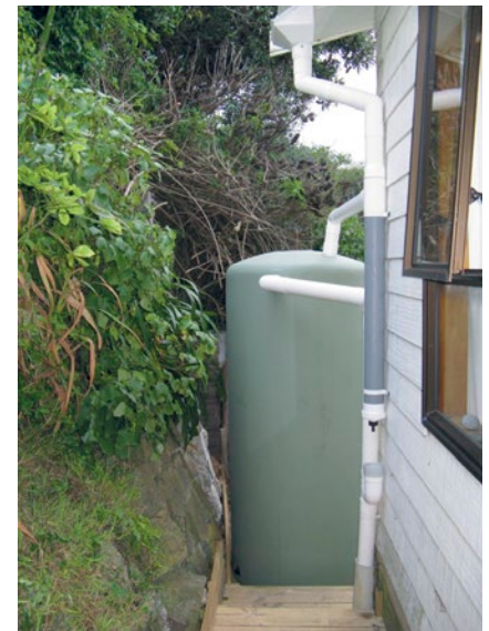
Fig 4: A 250 litre DEVAN rain water tank connected to down pipe via screened rain head and a 25 litre first flush diverter.
