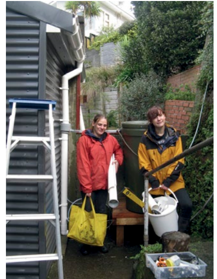
Figure 3: Mathilde Bertrand and Lucile Marsollier after installation of new gutters, downpipes, water diverter and 200 litre rainwater tank in Brooklyn.
