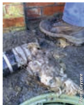
When disposed of into the sewer wipes bind together in a process known as ragging.
