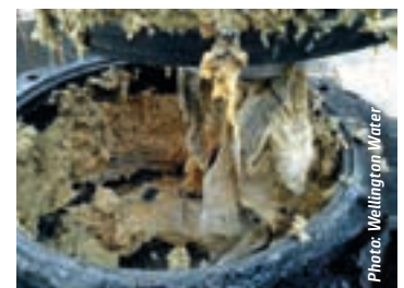
Wipes bound with fat and oil and grease being removed from a blocked wastewater pump station.
