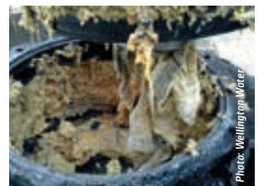
Wipes bound with fat and oil and grease being removed from a blocked wastewater pump station.
