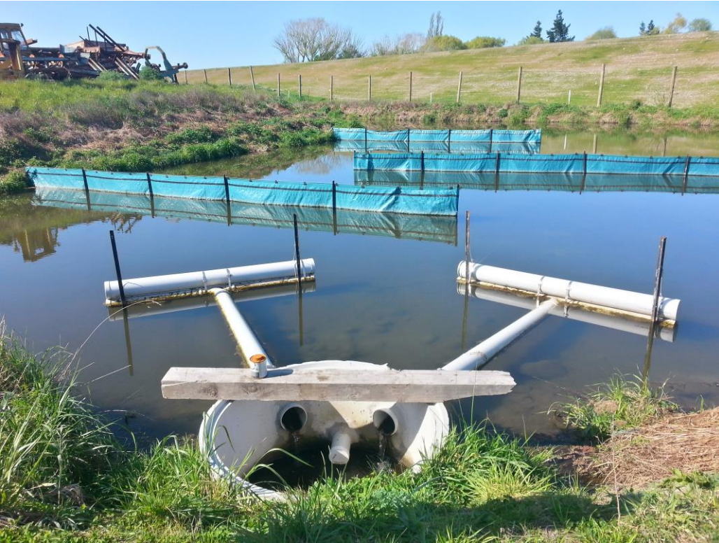
Figure 4 – The wetland in its temporary construction form with decanting outlet (this was the sampling point)
