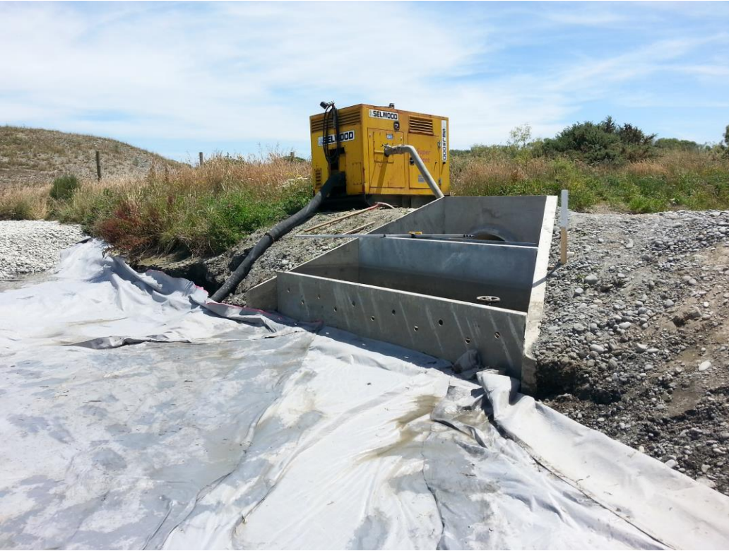
Figure 6 – Outlet headwall with baffle plate, screen and V-notch weir (obscured) under construction
