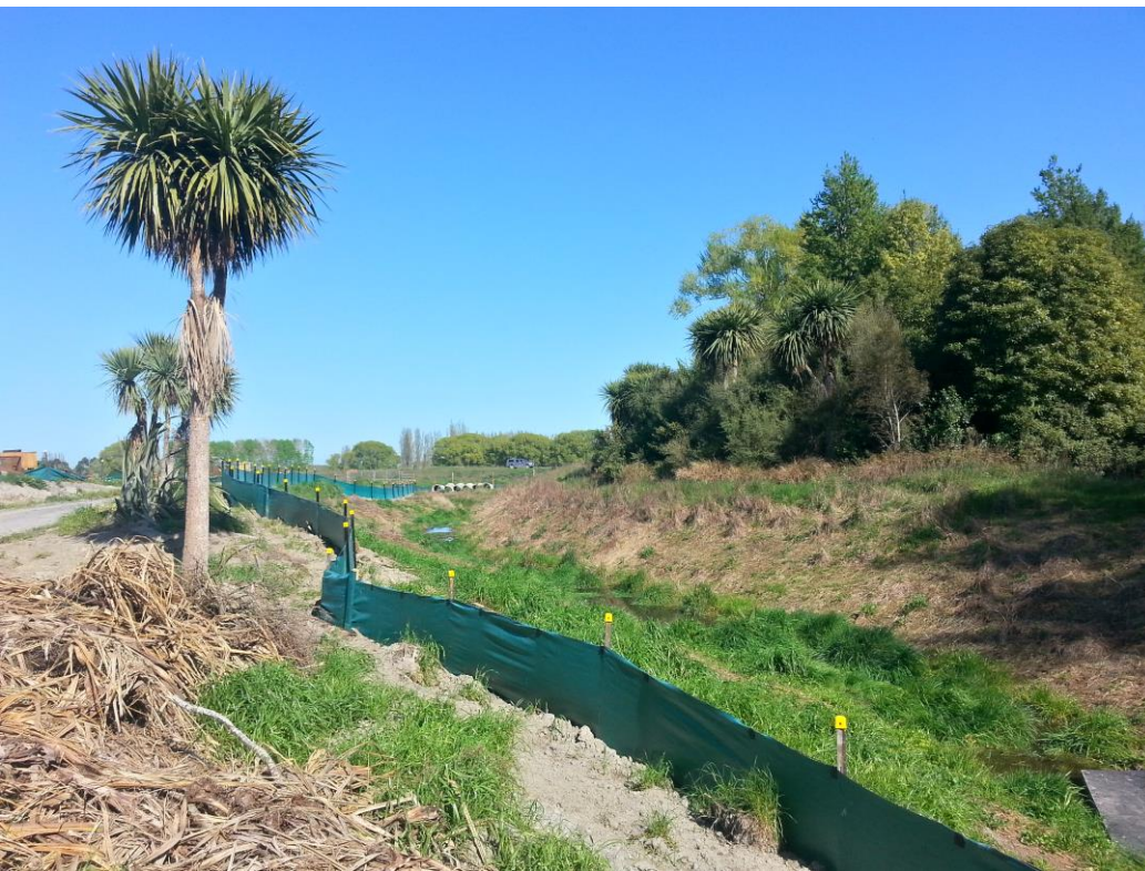
Figure 5 – The new outlet channel constructed to separate the discharge from the existing drain
