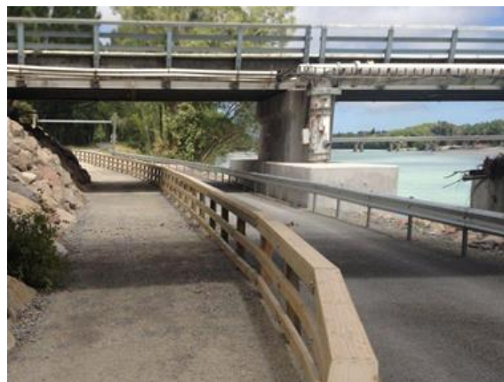
Figure 9: Separation of cycle way and road way at entrance to park on south side undertaken in conjunction with Rock Protection work
