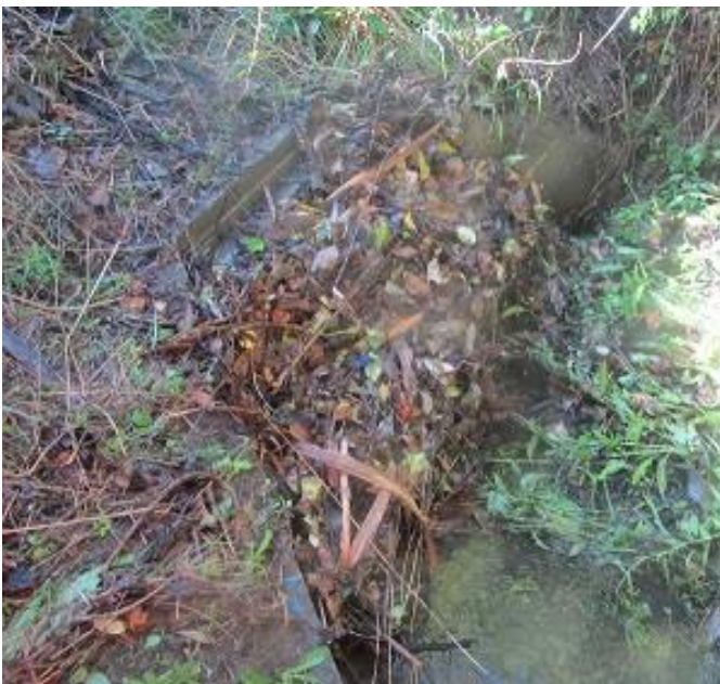
Photograph 2: Blocked Culvert Inlet
