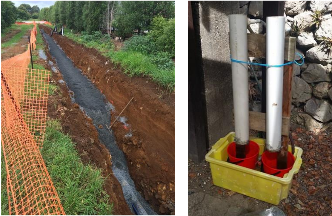
Figure 2: Rain garden during construction showing subsoil, drainage aggregate, and blinding. Percolation testing of rain garden material build up.
