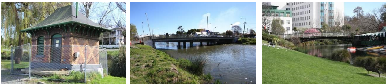
Photograph 4: Earthquake damage to a pump station and bridges in Christchurch
