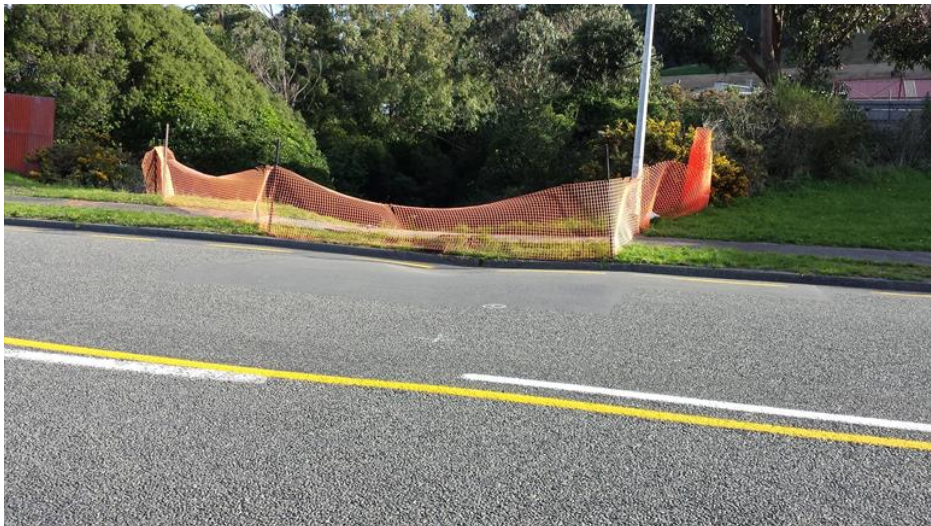
Figure 9 - Slumping of Raiha Street above culvert
