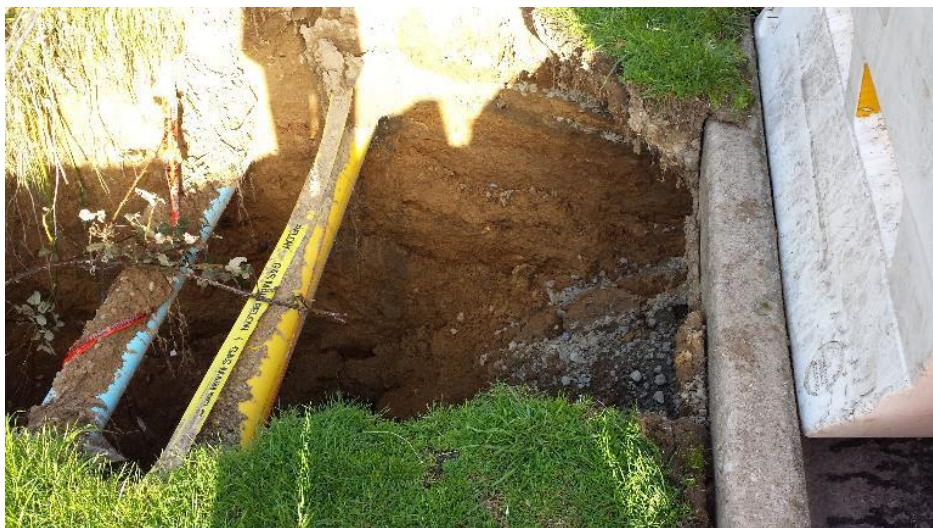
Figure 10 - Piping failure of embankment fill (downstream side)
