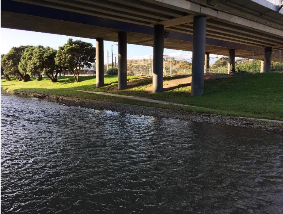
Figure 12 - Gravel build up to the top of the ~ 1 m high river bank walls in Porirua Stream
