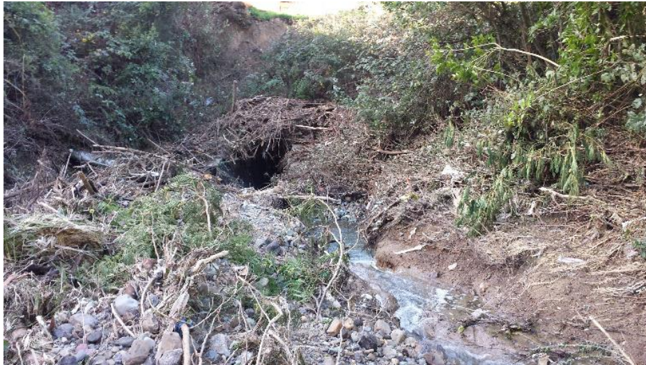
Figure 8 - Debris upstream Raiha Street Culvert – Mitchell Stream (post event)
