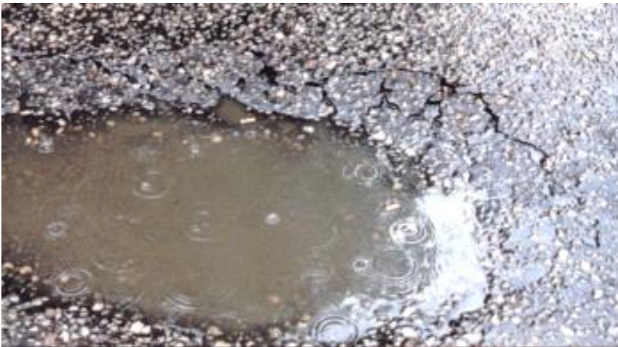
Figure 9 A pothole in caused by poor sub-base drainage.
