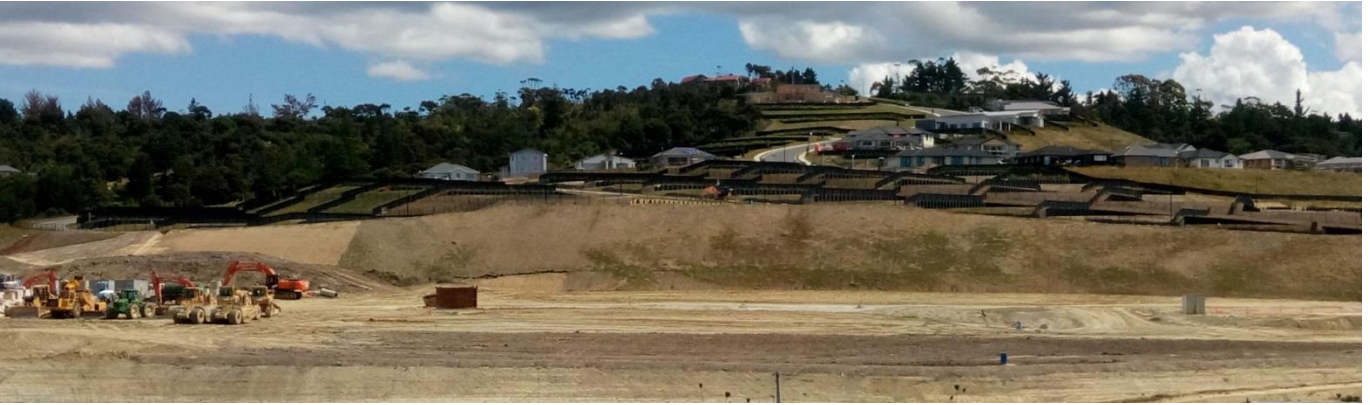
Figure 11 The Karapiro Drive development in Whangaporoa, note the numerous retaining walls and fleet of motor scrapers employed to create flat sections.
