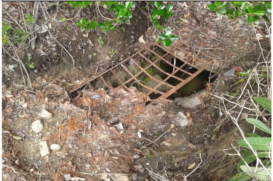
Figure 7: Case Study 3 – debris blocking inlets resulting in overland flow
