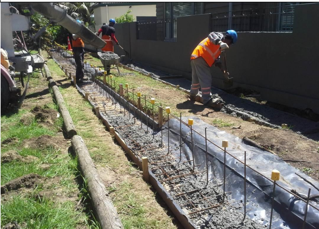
Figure 6: Case Study 2 – flood defence wall providing additional protection to property (currently under construction)
