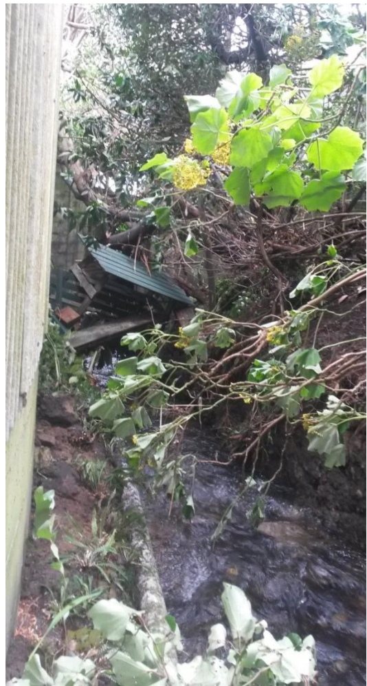
Figure 13 - Debris blocking open drains in private property
