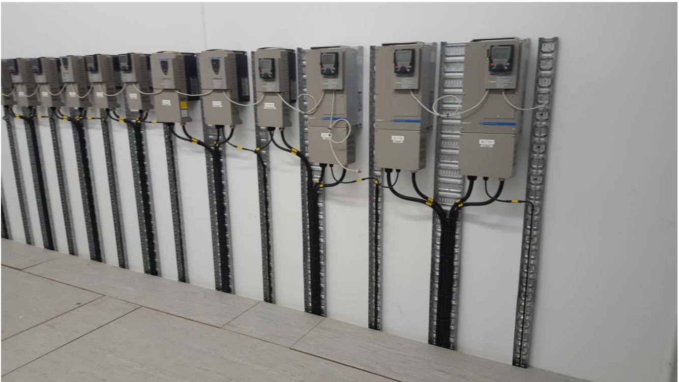
Photograph 1: Wall Mounted VSD's - note the break in the daisy chain
