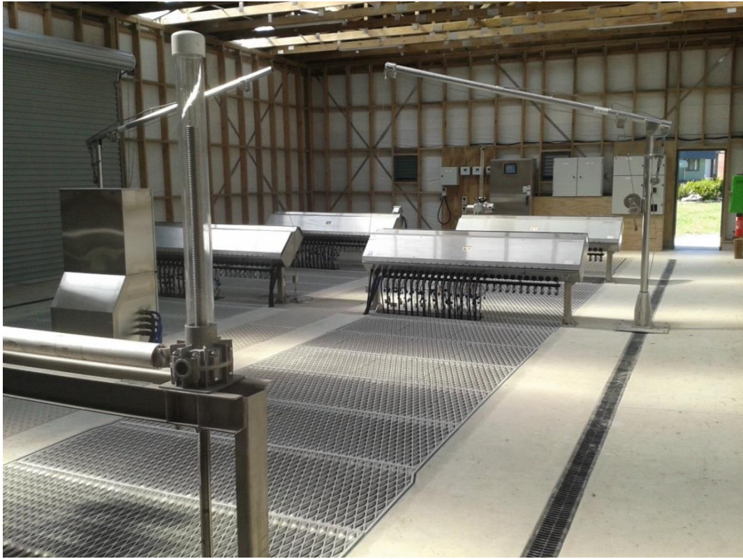
Figure 10 Whangarei Wastewater Plant Storm UV System
