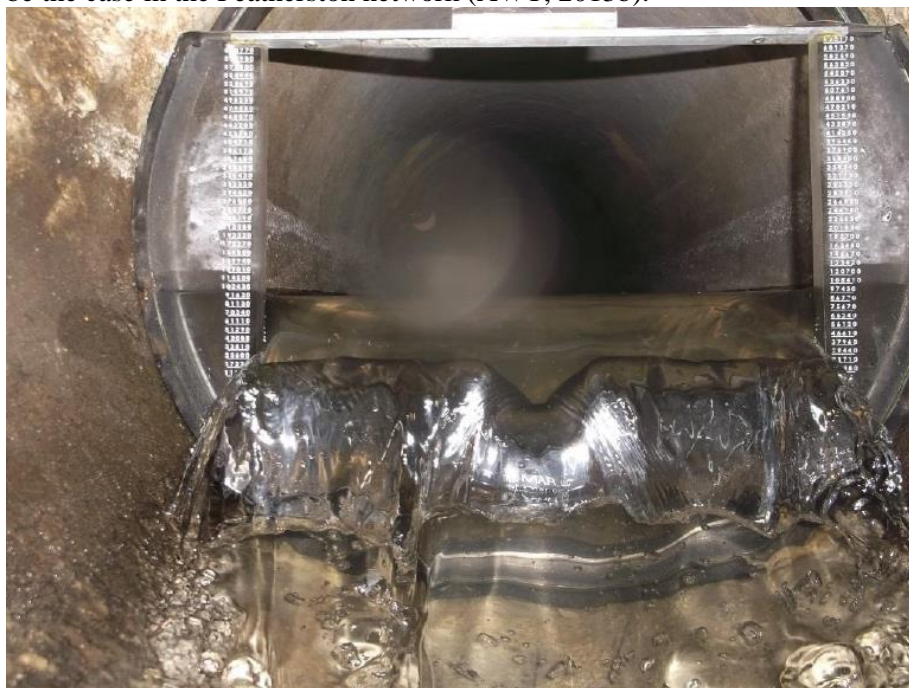
Figure 2: Night flows observed during night flow isolation I&I investigations in Featherston (note clarity of sewer flow)
