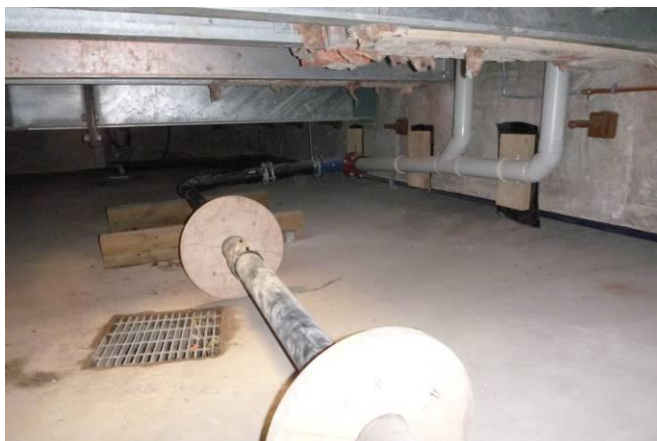
Photograph 6: Crèche Wastewater Connection
