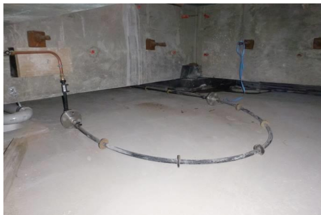
Photograph 7: Crèche Water Supply Connection
