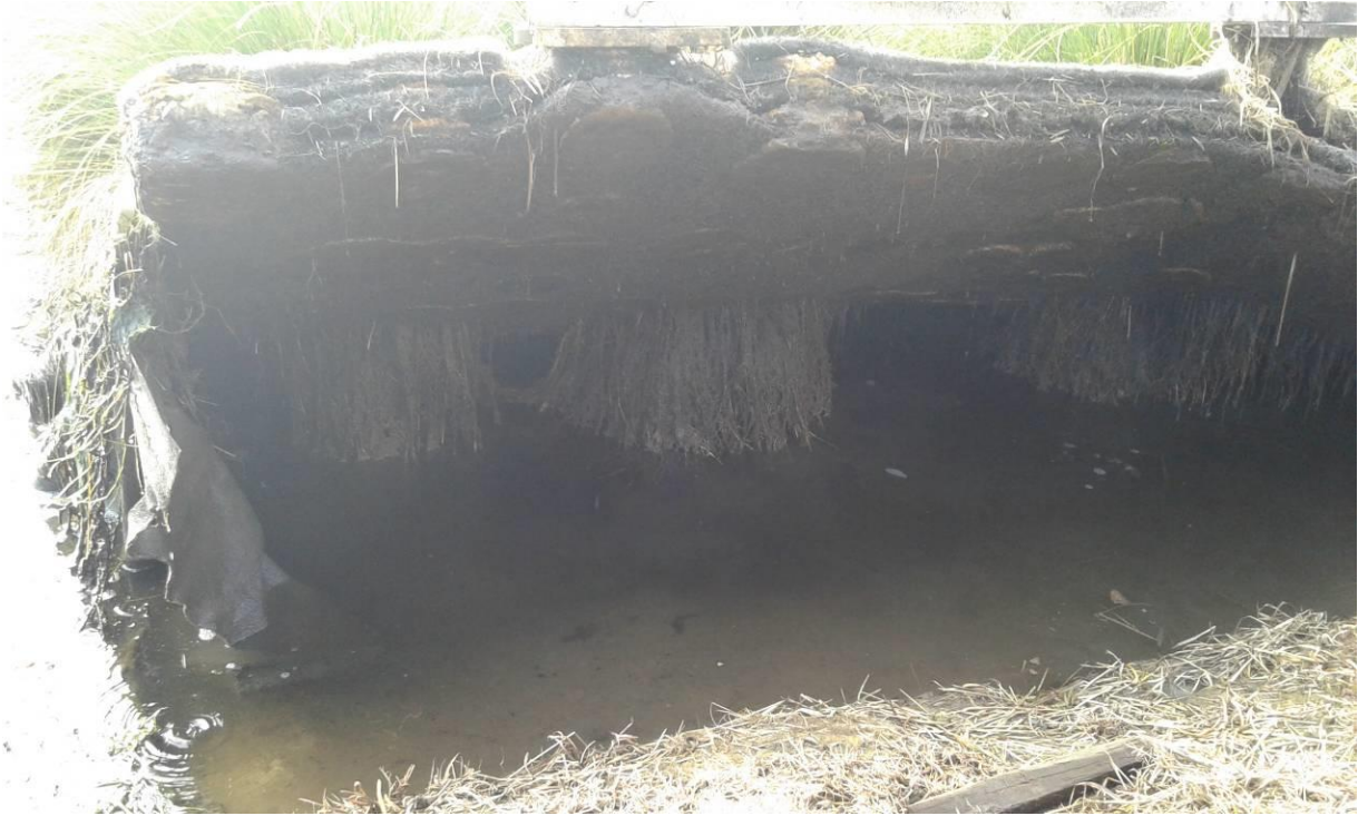
Photograph 4: Lifting of one of the floating pods close to the outlet of Kioreroa Rd WWTP wetland.
