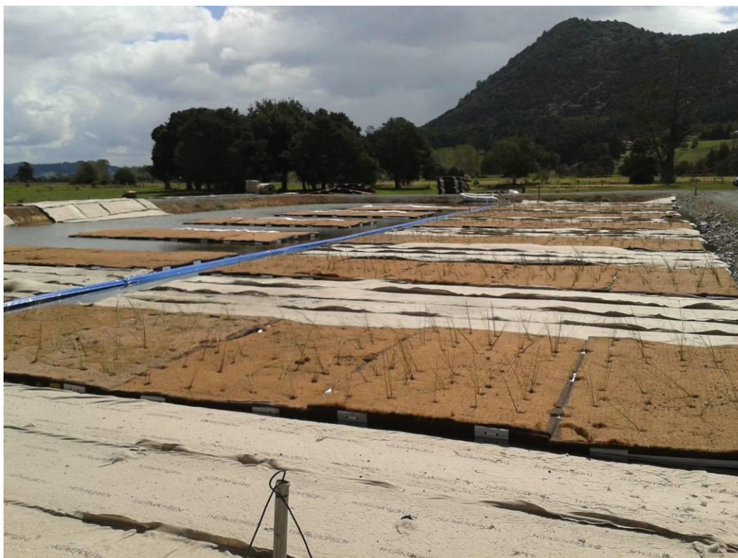
Photograph 5: Photograph of the newly installed and planted FTM wetland at Hikurangi WWTP.
