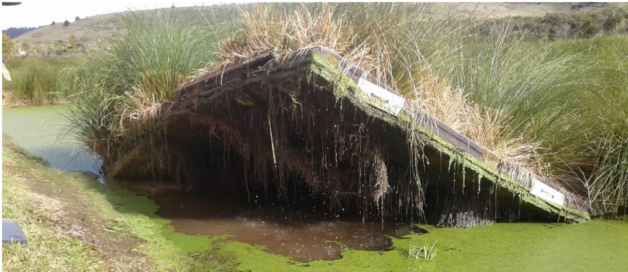
Photograph 3: Lifting of one of the floating pods at the inlet end of the Kioreroa Rd wetland.
