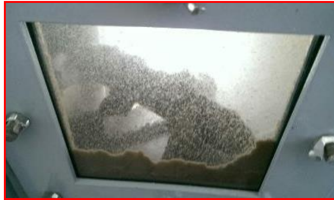
Photograph 5: Inspection Window at bottom of Settling Tank Showing Floc Formation and Sludge Scraper
