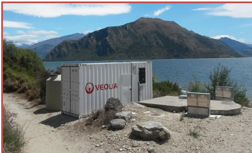
Photograph 4: Trial Unit Laydown Area showing the Plastic Sludge Tank
