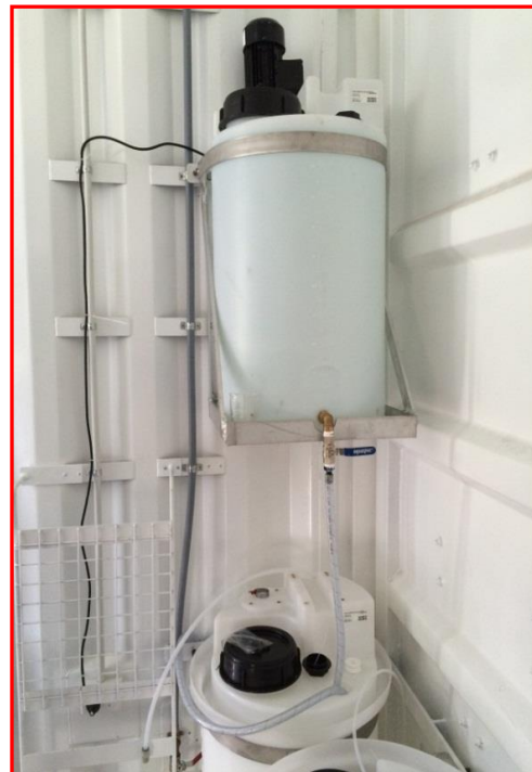
Photograph 3: Polymer Batching Tank
