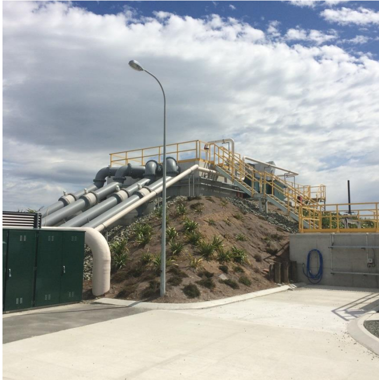
Figure 7: Domestic Inlet Screening Structure
