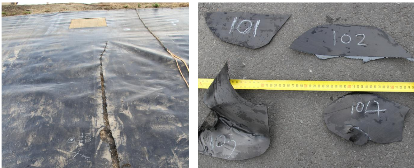
Photographs 1 & 2: Liner showing tear line, detailed damage of various areas and testing area
