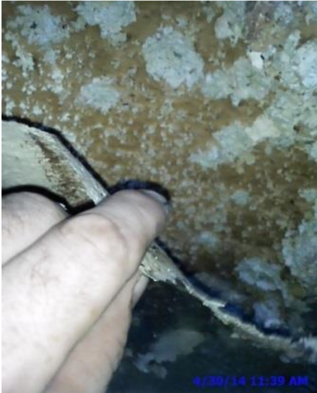
Photo 1 : Epoxy Coating (sheet) dislodged after 8 years at Manhole 0221
