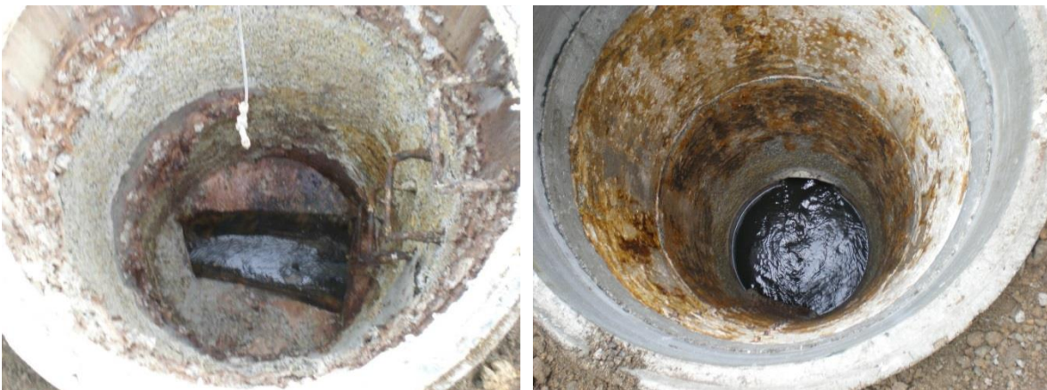
Photo 2: Continued Corrosion of Concrete & Steel Manhole 0226 & 0229.
