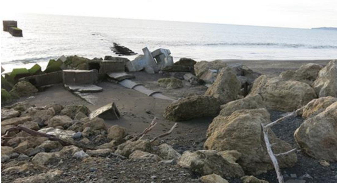
Photograph 1: Beach and Short Outfall – Damaged in recent storms
