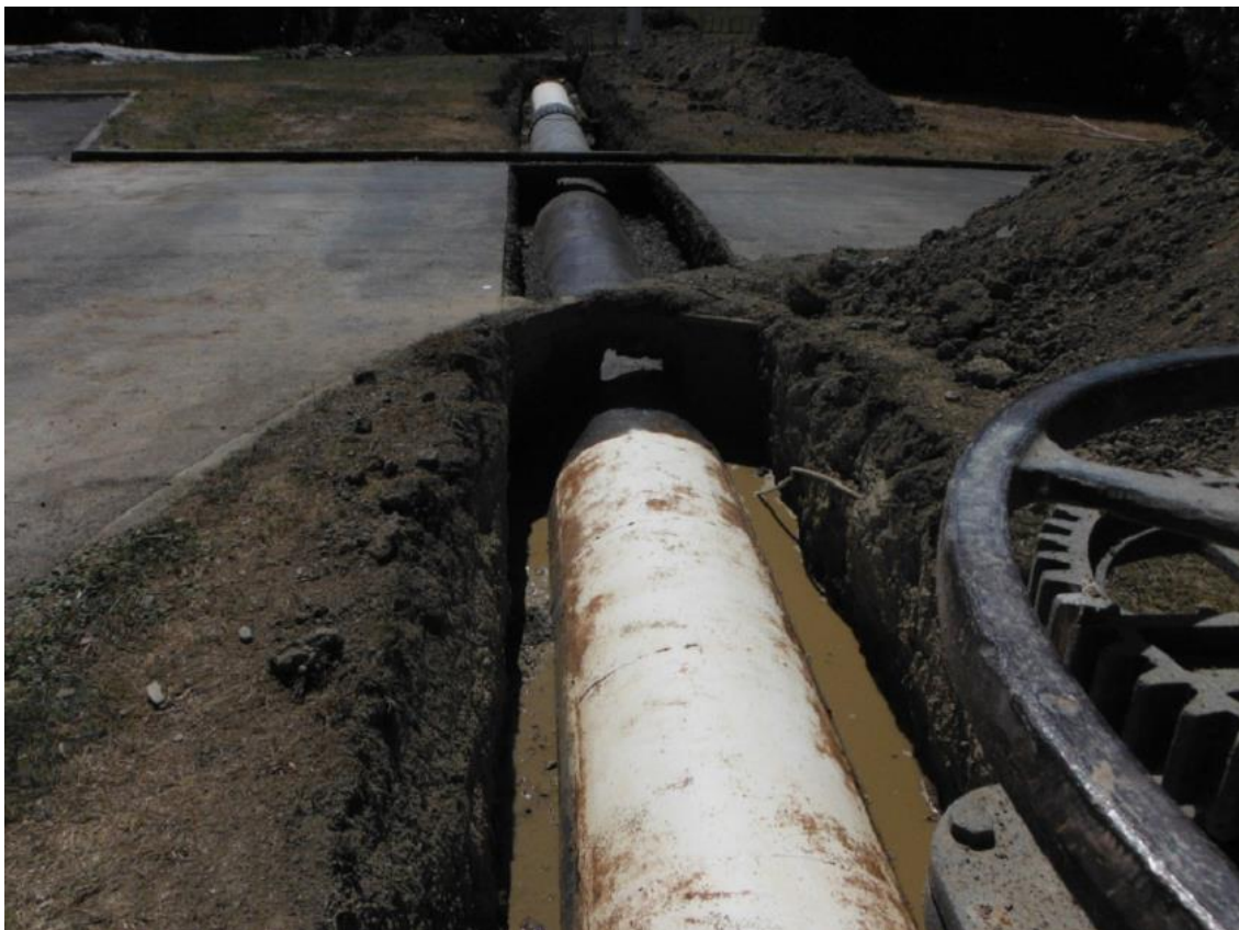
Photograph 3: Exposed Steel Pipeline
