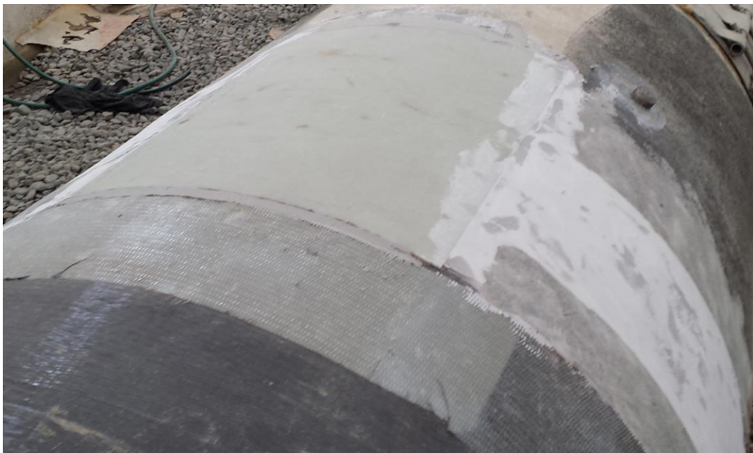
Photograph 5: GRP patch in area of “breakthrough” Corrosion at a Pipe Joint
