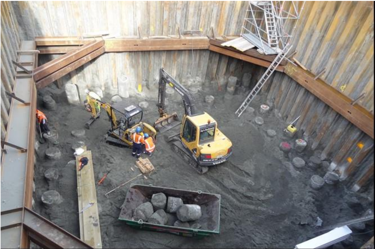
Figure 5: Construction work at the base of the wet well for PS 136, showing the tops of the 600mm-dia. CFA piles.
