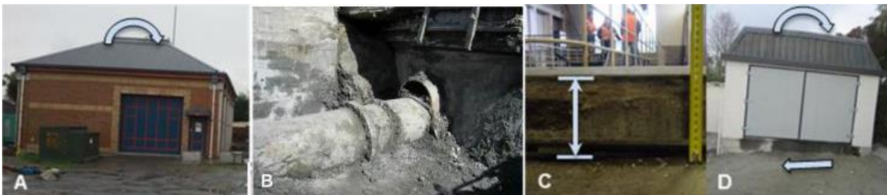
Figure 4: Common failure mechanisms at pump stations
