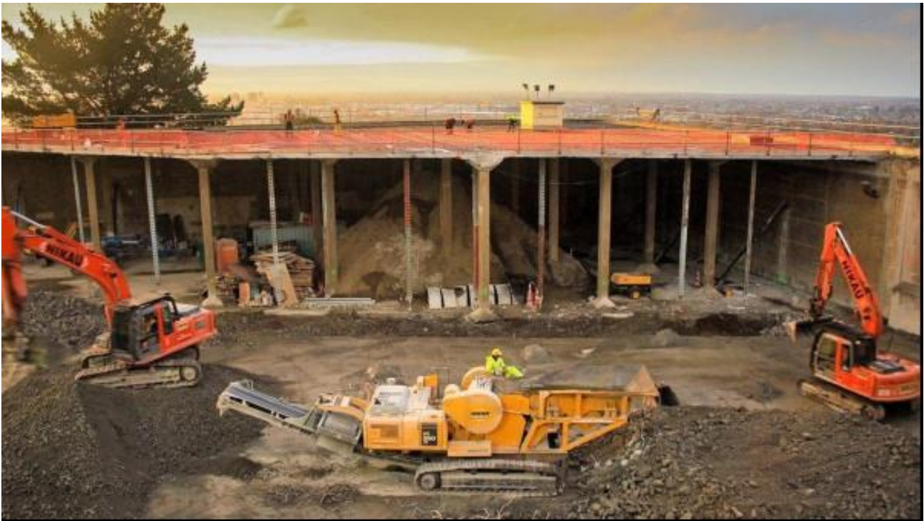
Figure 2: Construction activities at the Huntsbury Reservoir site in 2011, with machinery working in the area between the two halves of the 'new' reservoir.
