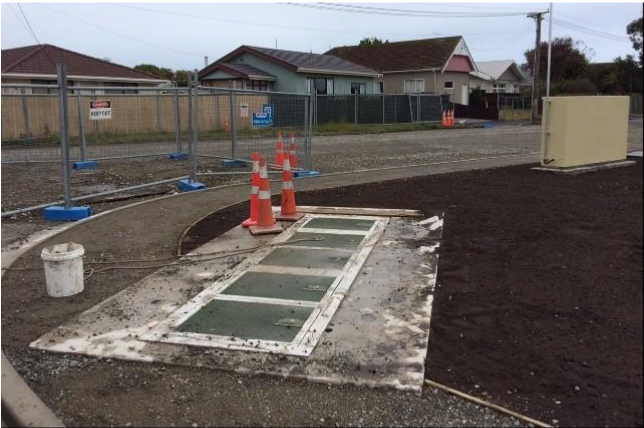
Figure 7: The near-complete horizontally-mounted PS 230 installed in the road verge at Owles Terrace.
