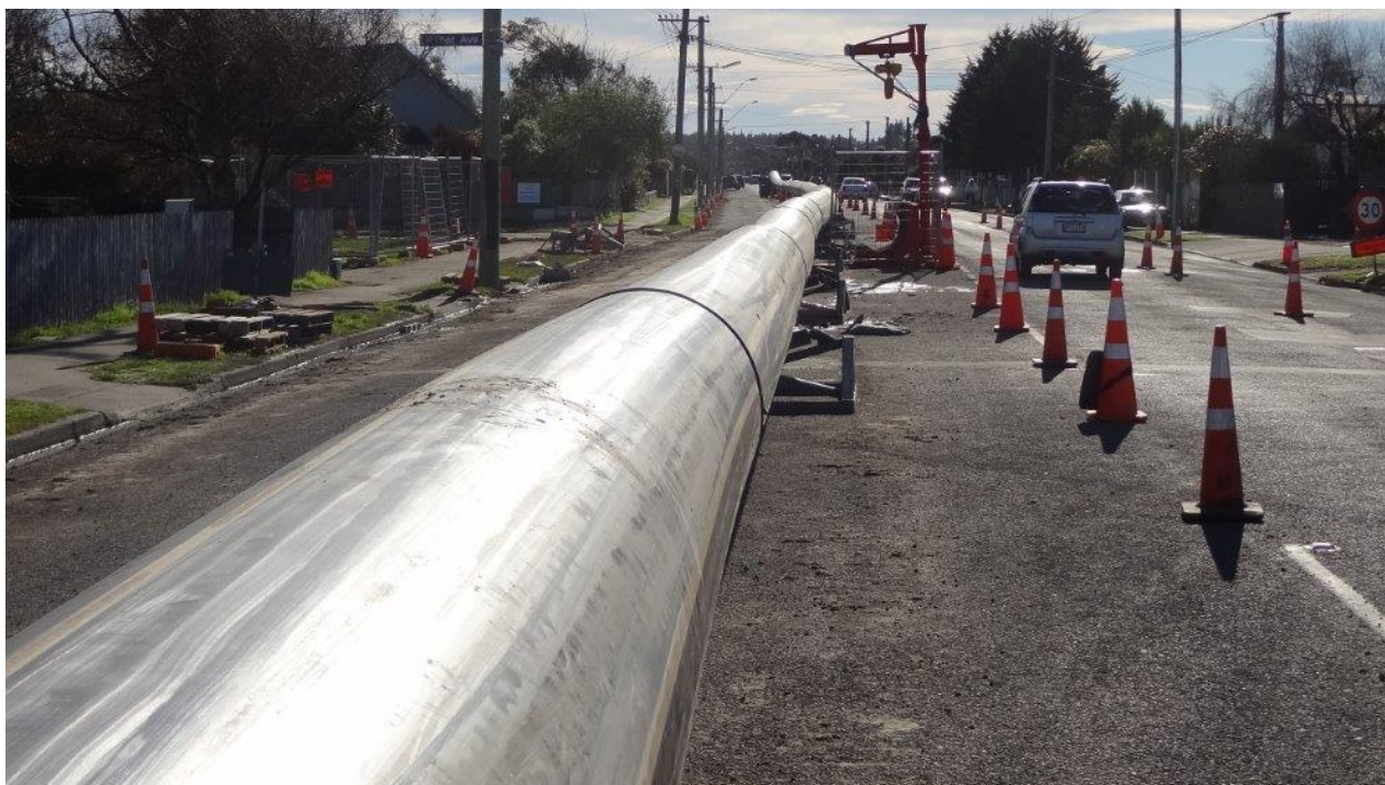
Figure 3: The DN800 PE PM 128 pipe running along Bower Avenue prior to installation by directional drilling.
