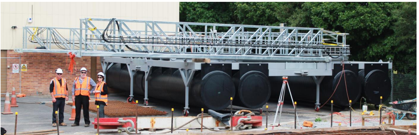
Photograph 3: City Waters staff and contractors with the barge platform after it was assembled at the Hamilton’s water treatment plant in January 2016, illustrating the scale of the pontoons.
