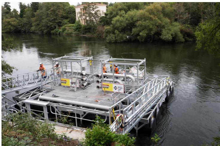
Photograph 6: The completed pumping platform awaits the installation of the suction hoses in February 2016.
