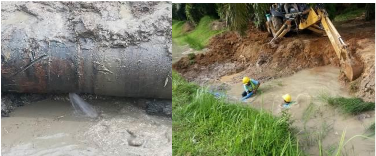
Figure 15: example of a leak in a buried water pipeline and the damage caused by a pipe burst
