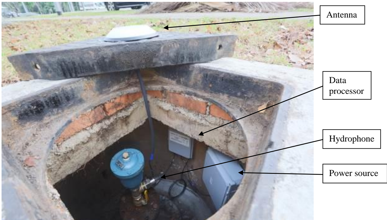
Figure 12: An example of a node installed in an existing air valve chamber
