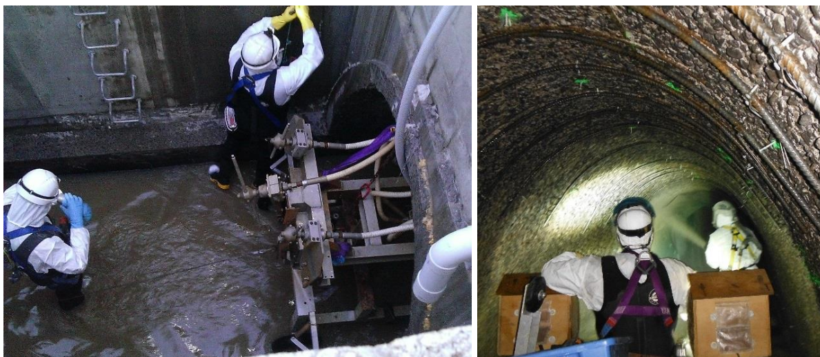
Figure 8. Remote cleaning unit modified for the elliptical pipe section (left), and wheeled work trolley with SewperCoat® application in the Sylvia Park section (right)
