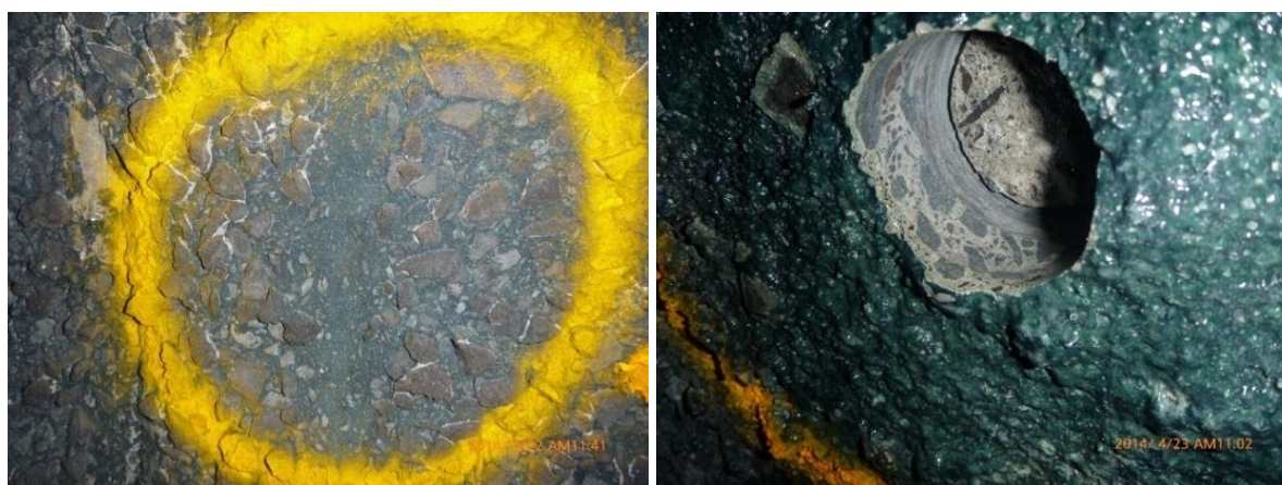
Figure 9. Black organic staining which appeared on alkaline surfaces of cleaned concrete and applied SewperCoat® in SP2
