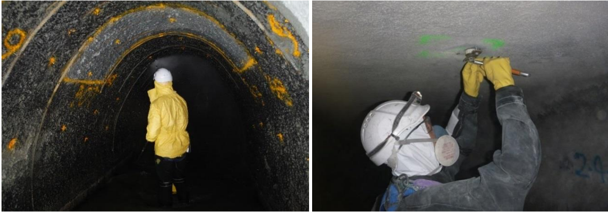
Figure 6. Inspection following hydro-demolition and rebar installation in SP2 (left), and SewperCoat® adhesion testing (right)
