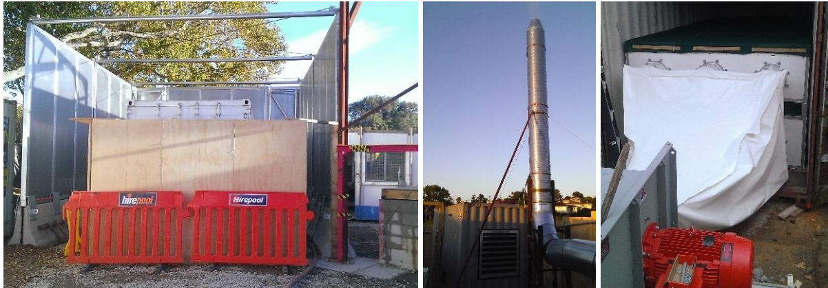
Figure 10. Noise control enclosure in Sylvania Park School (left), ventilation chimney (centre) and activated carbon filter for odour control (right)
