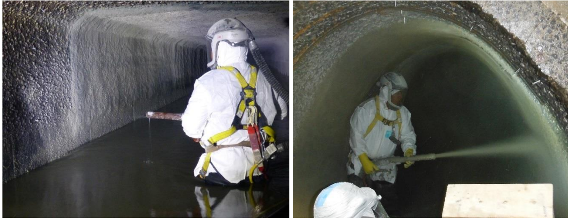
Figure 2. Internal profiles of the Eastern Interceptor and typical equipment for gunite application in the Eastern Interceptor
