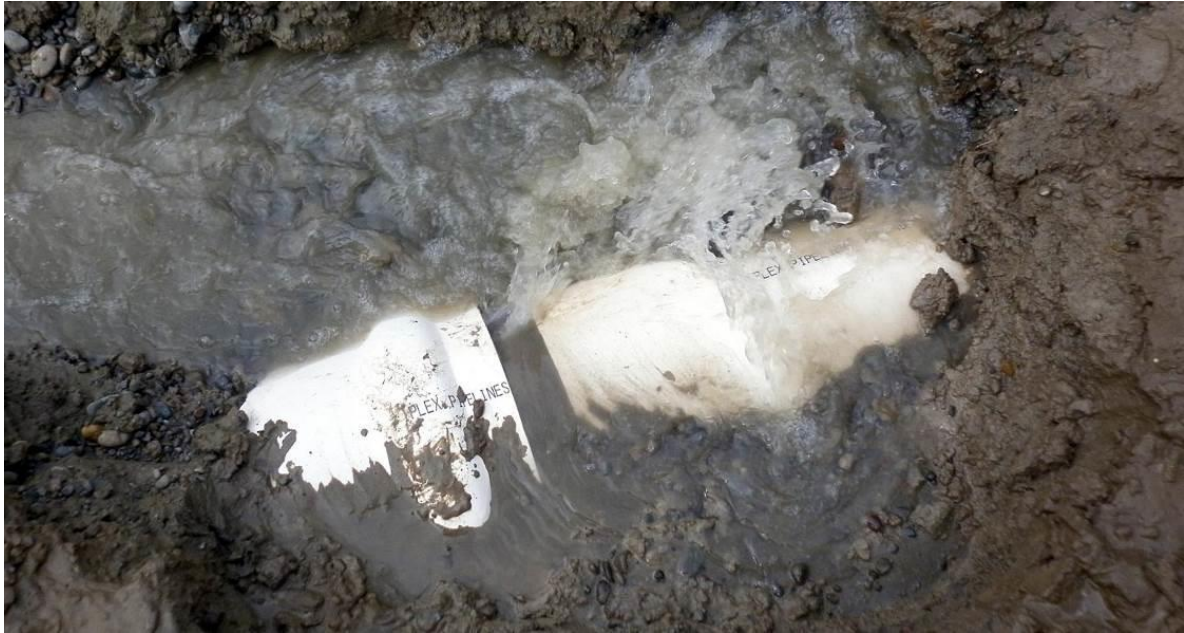
Photograph-2: View of the joint pull-out and leak that occurred as a result of the September 2010 earthquake (Photo - Gary Boot WDC)
