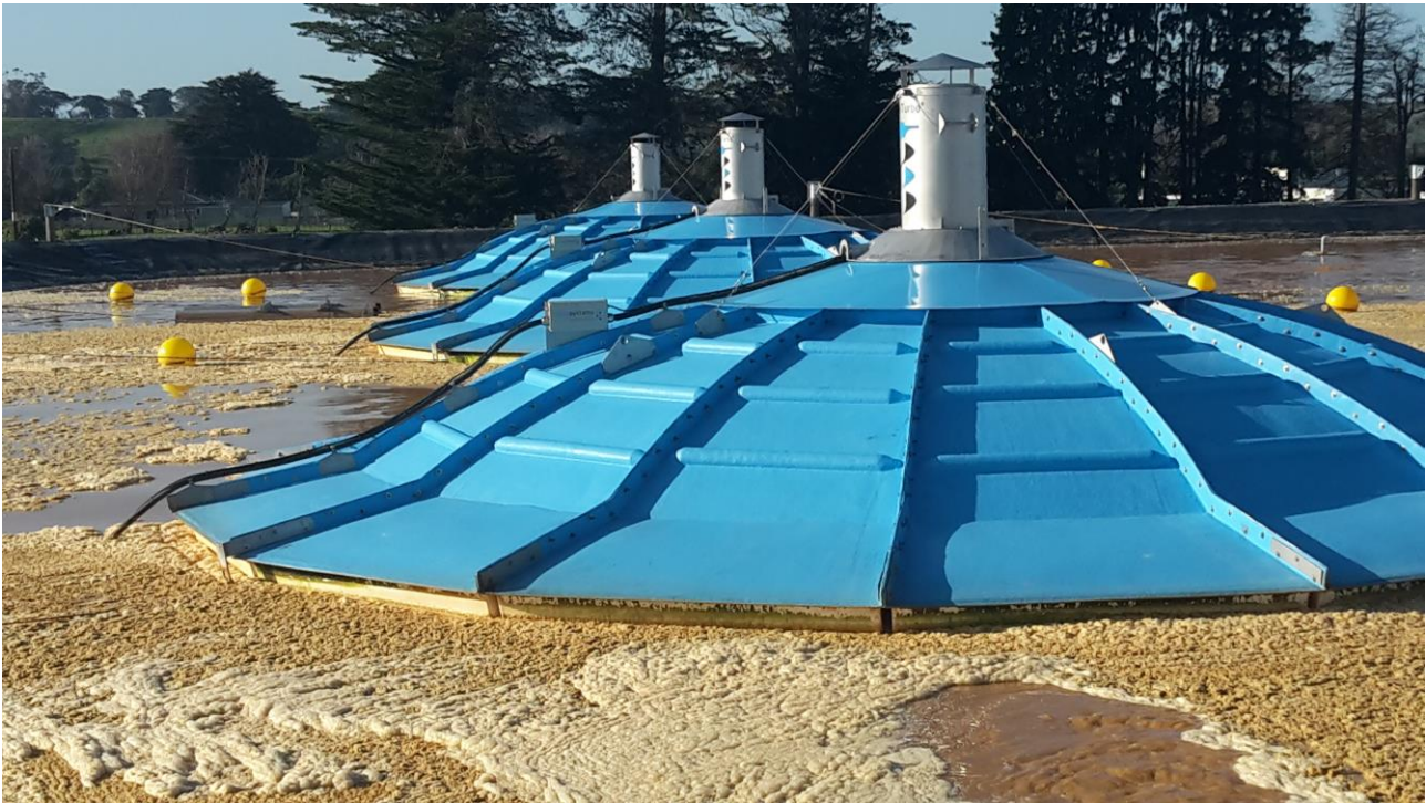
Figure 2: Floating Surface Aerator with Acoustic Cover and Motor Silencer
