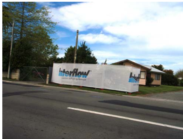
Figure 8. The footprint of the Rehabilitation of No.3 Trunk Sewer in Hastings, 628m of 1.8m diameter using Interflow's Rotoloc spiral wound lining technology.
