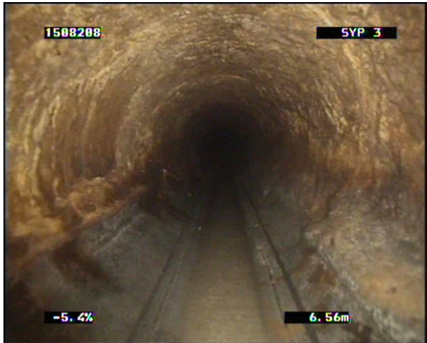
Photograph 4: Corrosion on the descending leg of one of the siphons
