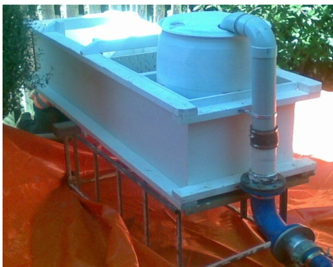
Photograph 2: The weir box flow measurement device discharging to a local manhole
