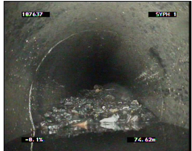
Photograph 5: Silt build up at the transition from horizontal to ascending leg
